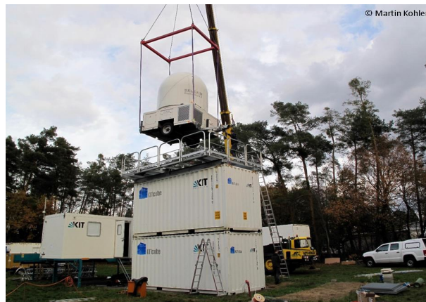
Installation of the x-band rain radar on top of a tower consisting of two transport containers. Test setup at KIT in Karlsruhe, Germany.
